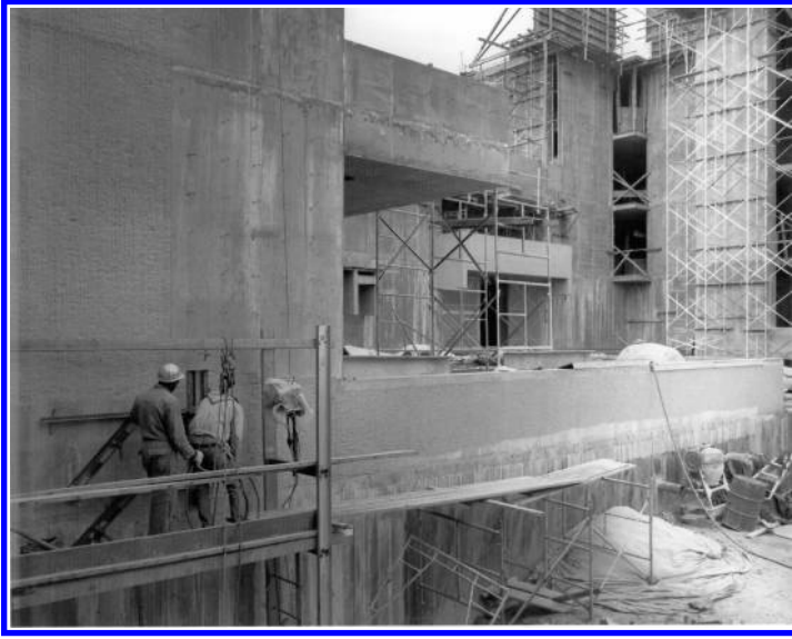
FIG. 3 NCAR's Mesa Laboratory under construction. Workers at the lower left are bush hammering the concrete for a uniform texture. Compare finished concrete with rough form finish to the right. Source: Martin Eby Construction.
